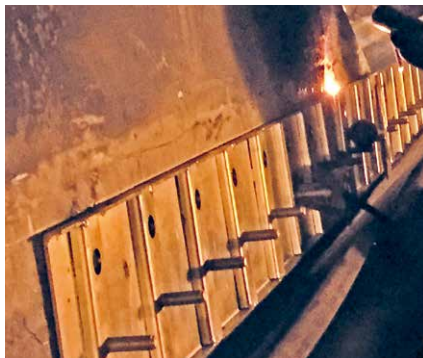
The first trial run of the FD side sealing system on a 1,600-mm-wide conveyor belt in a feeding tunnel with six loading points.
