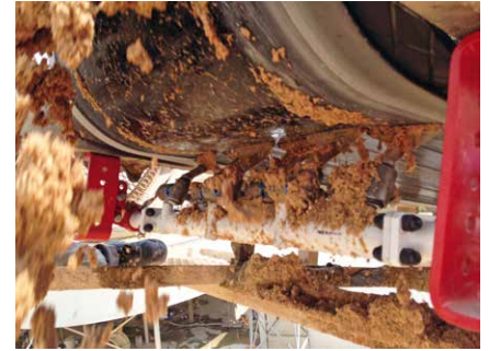
Gritty work: The HOSCH scraper on one of the 50 belt conveyors.
