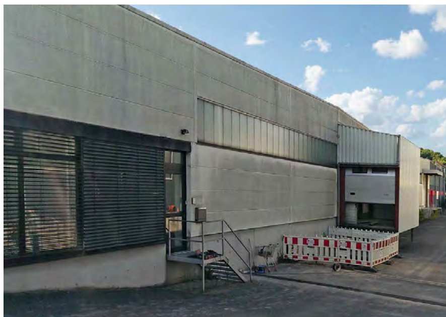
After extensive conversion work (including a new ramp for easy loading and unloading), HOSCH will be able to move into its new hall in late June.
