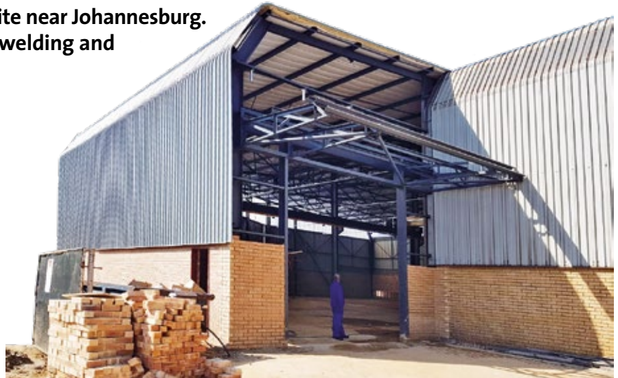
The addition of a new annex has created approx. 1,000 square meters of space for HOSCH South Africa. The project is expected to be finished in January 2021.
