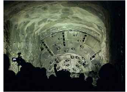
The breakthrough after almost five years: “Big Becky” finally sees light at the end of the tunnel; Photo: www.niagarafrontier.com
