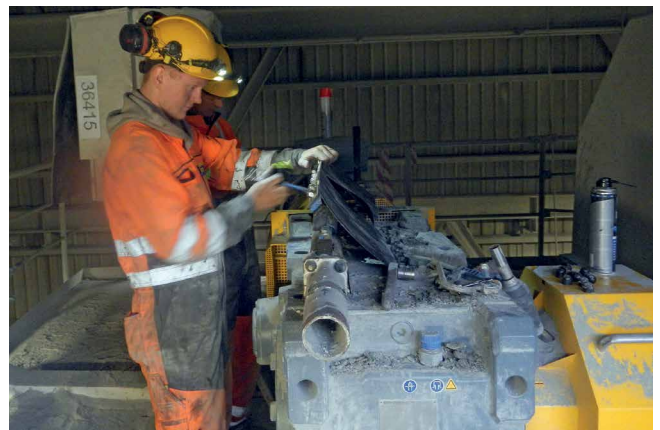
Installing a Type B6 scraper in the quarry at Norsk Stein A/S.
