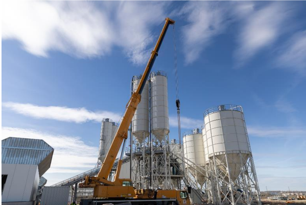
Concrete batching facility
