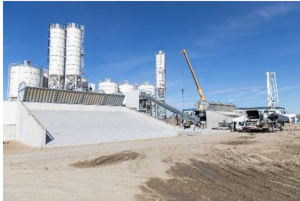
Concrete batching facility
