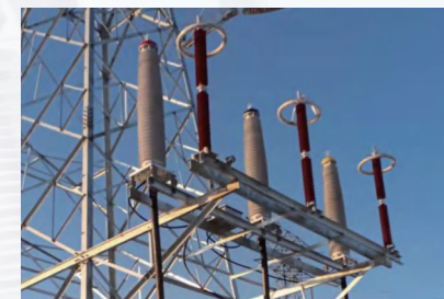
Sichuan Shanshan 220kV Transmission Line Project
