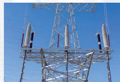
Yanggao 220kV Substation Project
