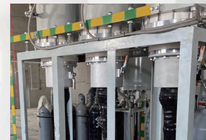
Phase I of Longma Wind Energy 220KV Substation in Tongliao City
