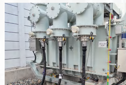
Yan'an Ansai Thermal Power Plant Cogeneration Project (Start-up/Standby Transformer)
