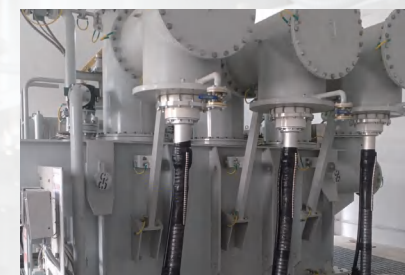
Shanghai Electric No.1 Main Transformer Project
