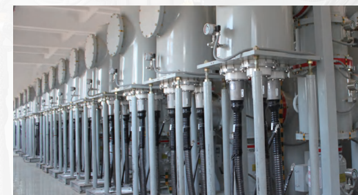
110kV Zongheng Group Fengnan Iron and Steel Project
