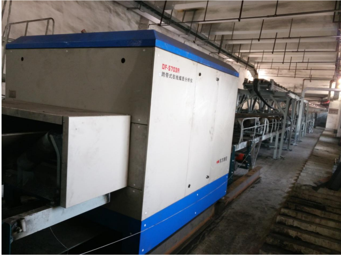
Fushun Ore Zhongji Thermal Power Co., Ltd.
